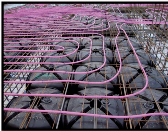
Warm or cooled air is pumped through pipes in the high thermal mass flooring to deliver heating and cooling for the school.
