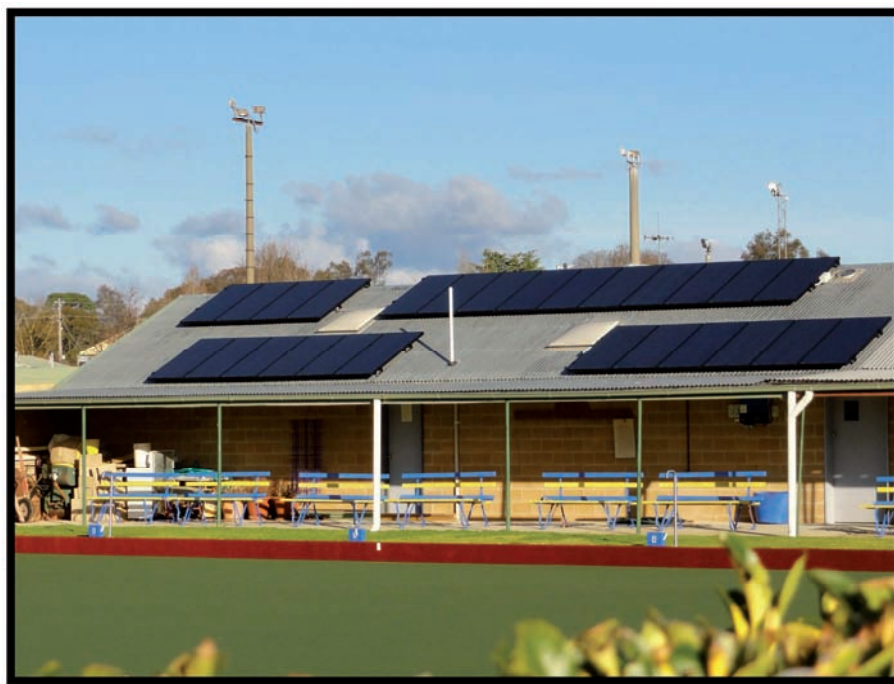
A 4.94 kW solar PV array was installed at Kiewa Bowls Club, Tangambalanga in June 2012. The system will be used to reduce consumption of grid electricity for Coulston Park user groups.
