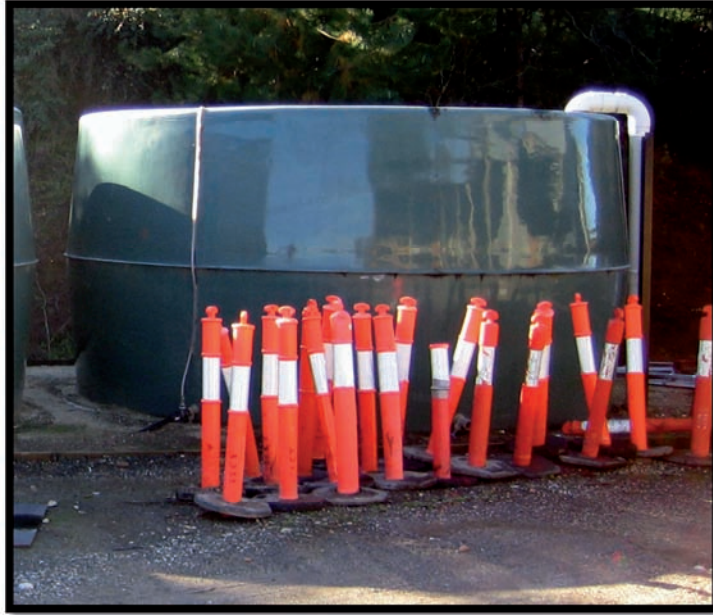
Water from this tank installed at Indigo Shire Council's Yackandandah depot is used to clean machinery.
