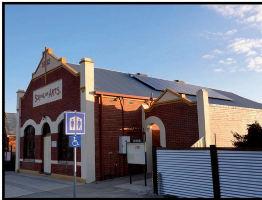
A 4.5 kW solar PV array was installed at the Wahgunyah School of Arts to help meet the electricity needs of the many community groups that use the facility.
