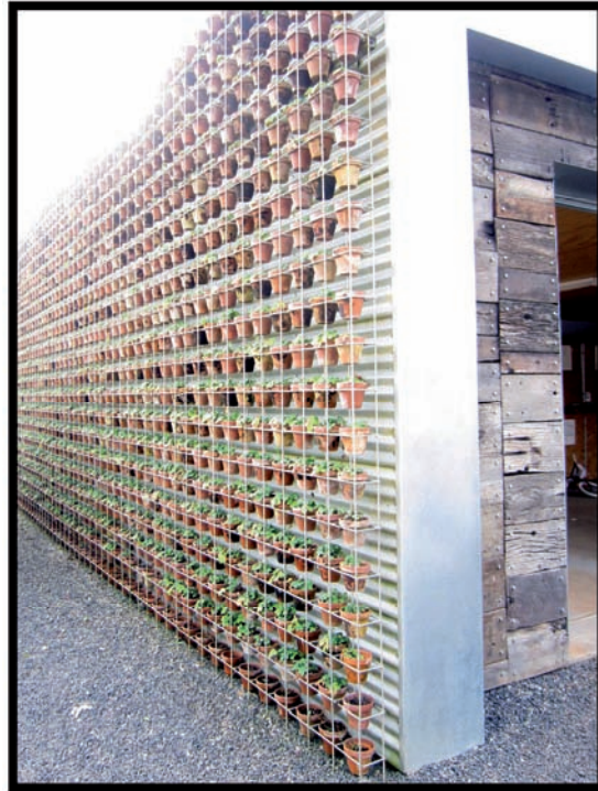
A vertical green wall of pot plants has been externally fitted to this building. It reduces radiant heat gain, improves insulation and in this case even provides produce.
