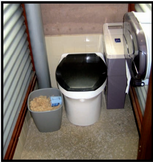
A waterless composting toilet at Charles Sturt University, Albury-Wodonga. Wodonga.
