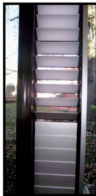
Louvre windows at Wangaratta's Performing Arts Centre are used to provide natural ventilation. The windows are connected to the Centre's heating and cooling to eliminate energy waste when open.
