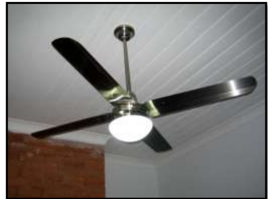
Figure 6: Install ceiling fans to offer air movement and cooling.
