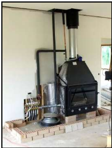
Figure 11: Slow combustion wood heater installed to act as a heat source and wet back boiler.
