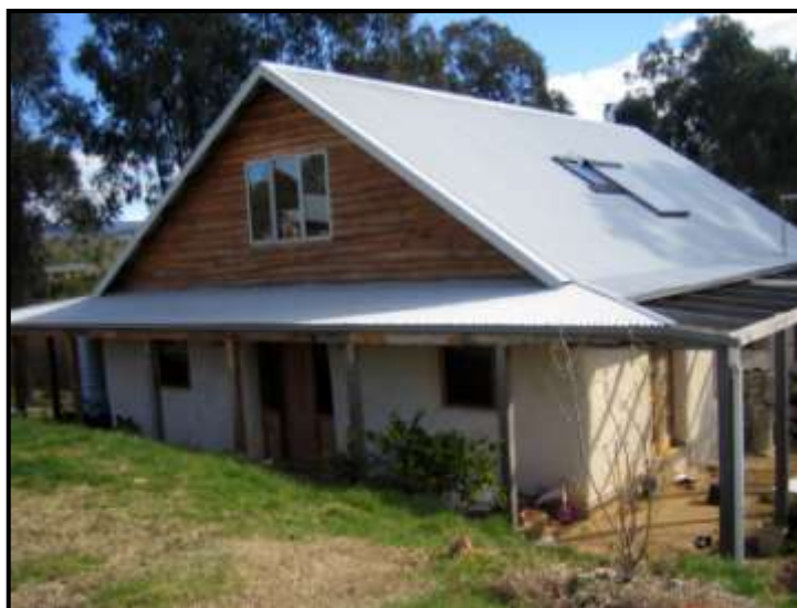
Figure 26: The thick straw bale walls of this home have been covered with an earthen render to seal and protect the building material.
