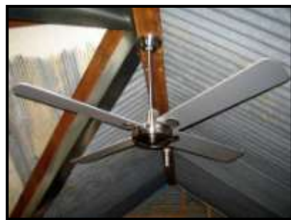
Figure 12: High level ceiling fan
