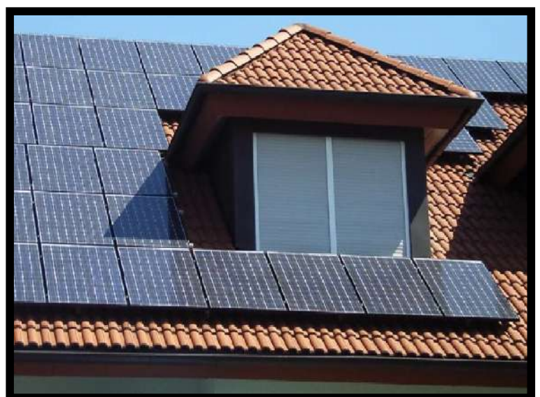
Shading of panels from the projecting roof line will affect the system's generation capacity.
