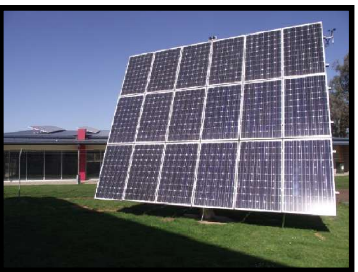
Sun tracking 4.3kW system installed at Wangaratta's Eco Living Centre.
