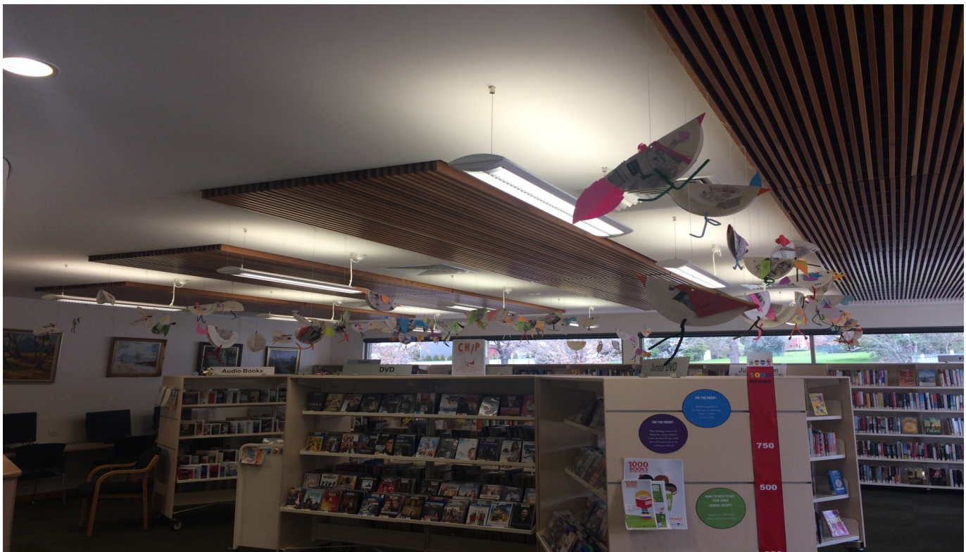
Photo: Energy efficient lighting at Yackandandah library
